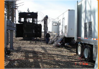
REGEN PROCESSING LARGE TRANSFORMER
